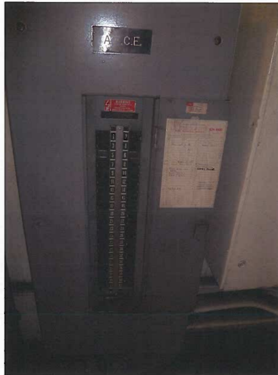
EXISTING PANEL "AFCE"
