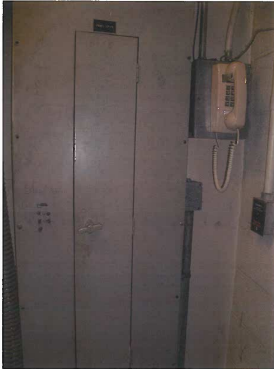
EXISTING PANEL "LP-FS"
