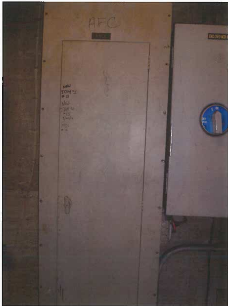
EXISTING PANEL "MNCC"
