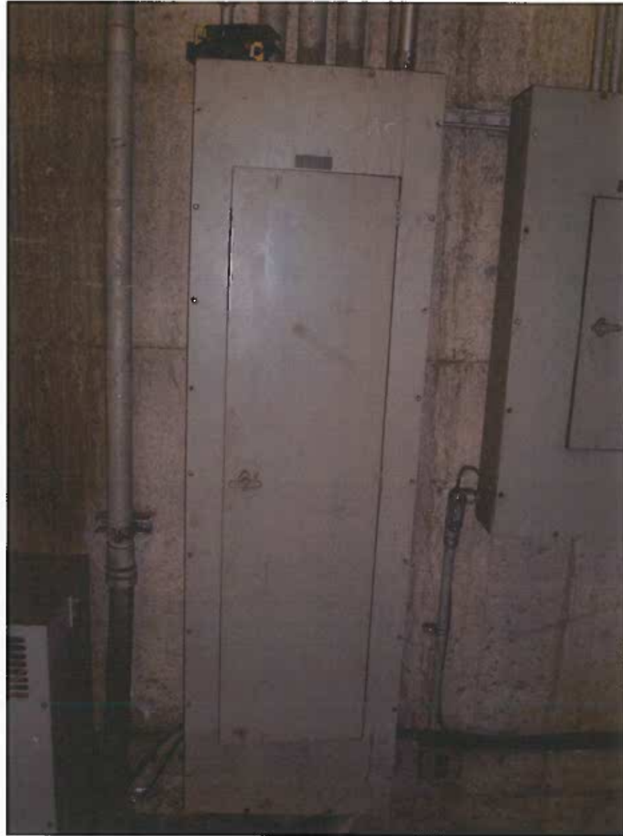
EXISTING PANEL "MSAA"
