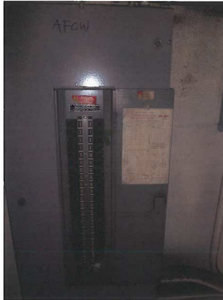
EXISTING PANEL "AFCW"
