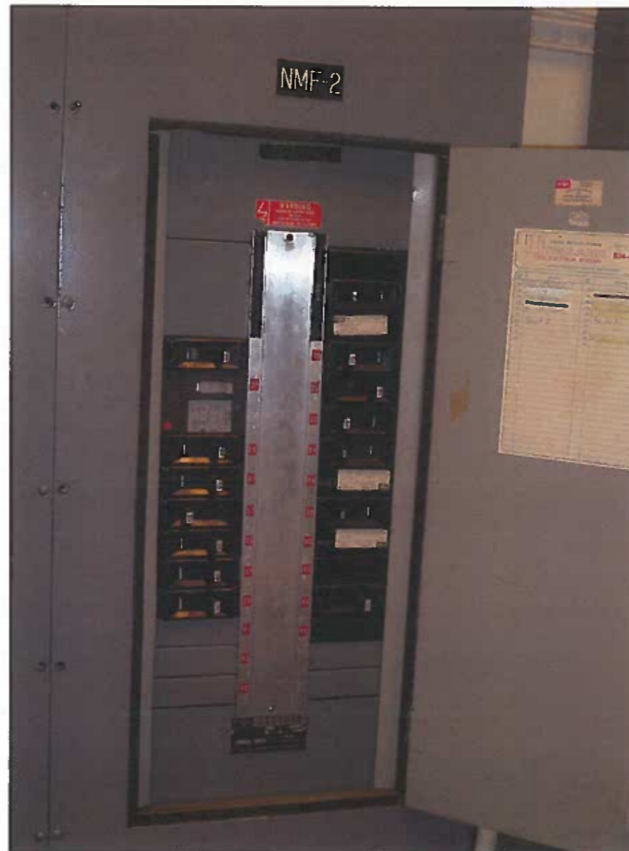
EXISTING PANEL "NMF-2"
