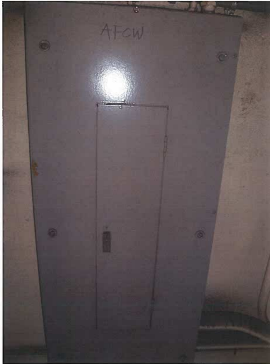
EXISTING PANEL "AFCW"
