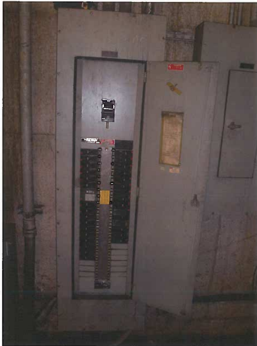
EXISTING PANEL "MSAA"
