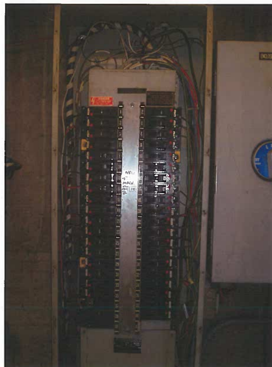
EXISTING PANEL "MNCC"
