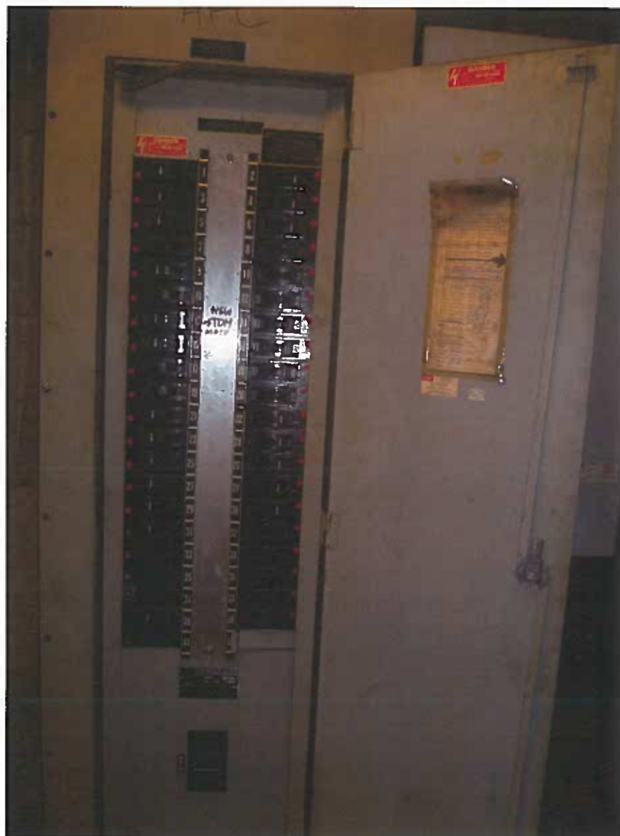
EXISTING PANEL "MNCC"
