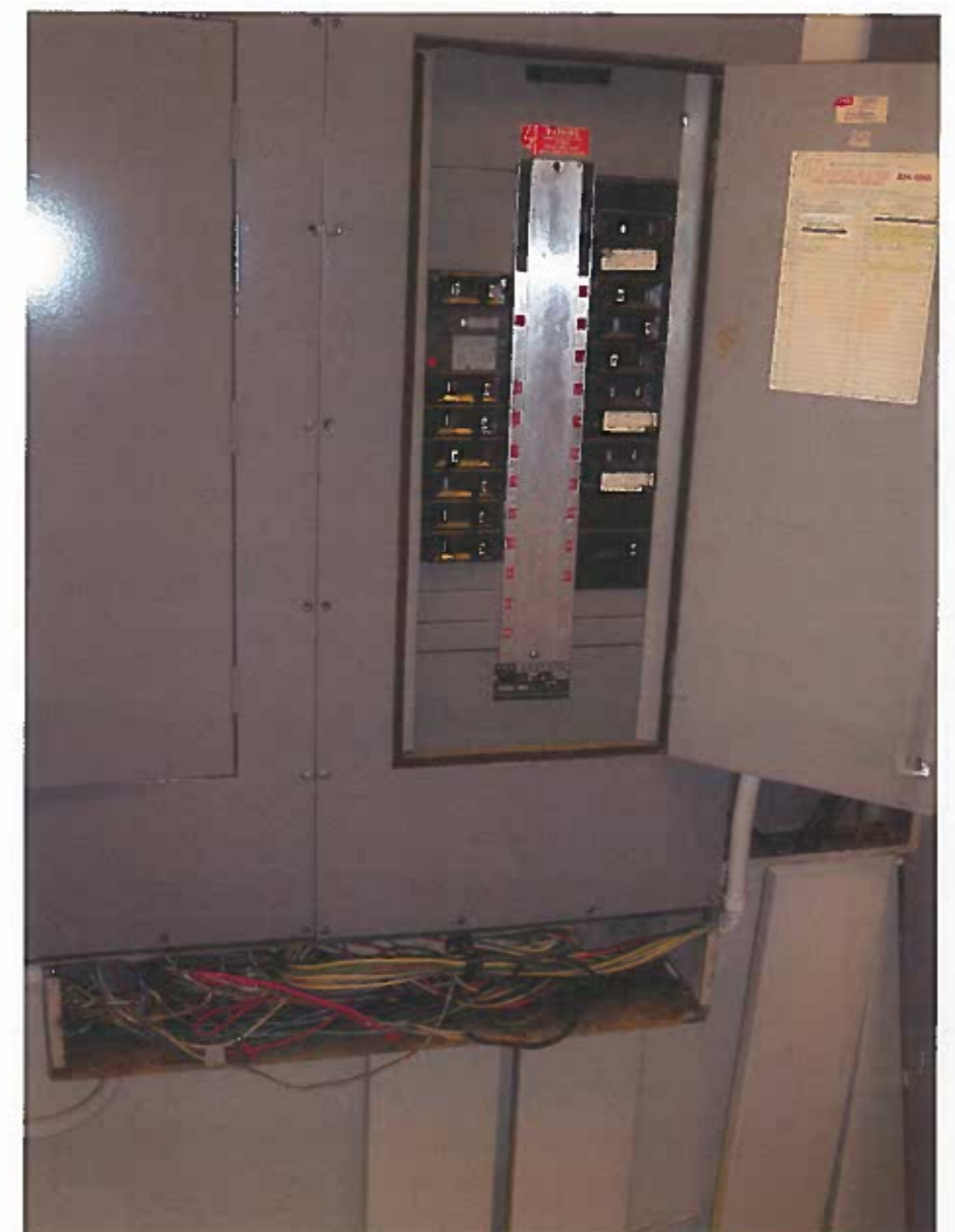
EXISTING PANEL "NMF-2"
