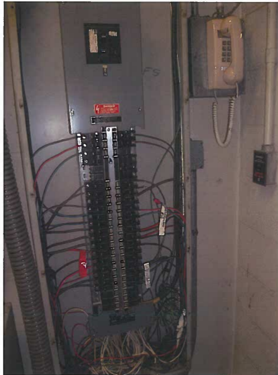
EXISTING PANEL "LP-FS"
