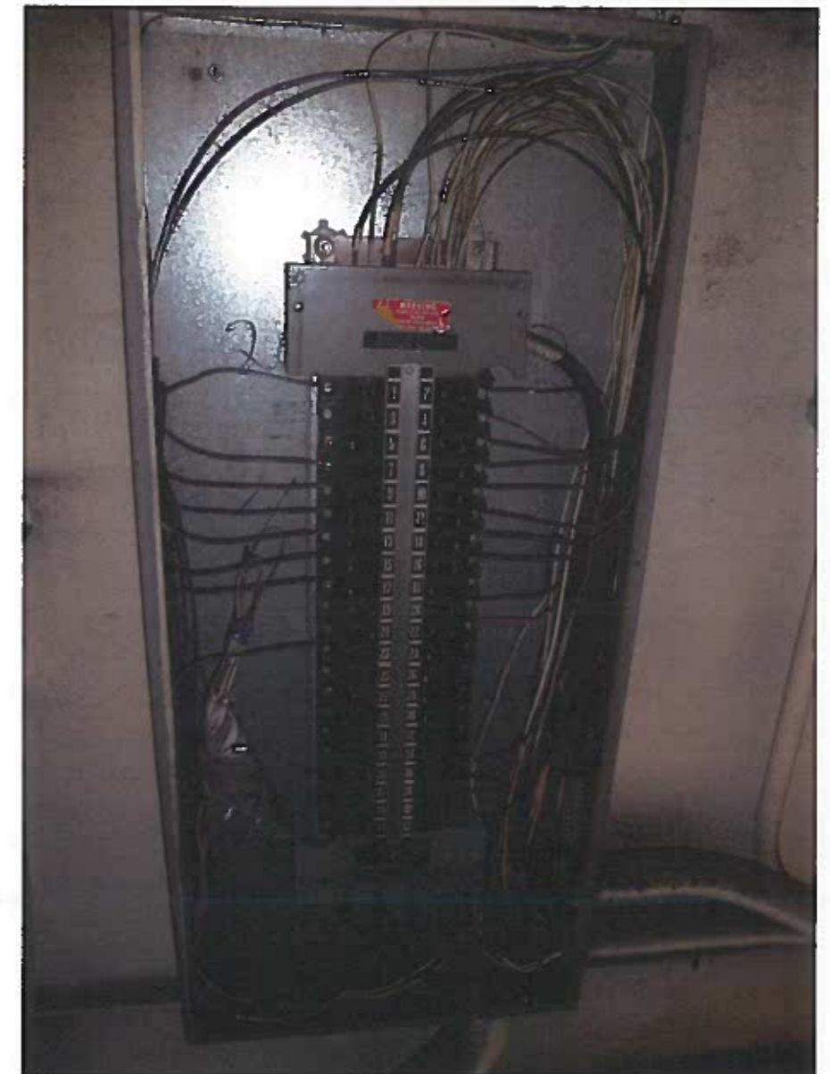
EXISTING PANEL "AFCW"
