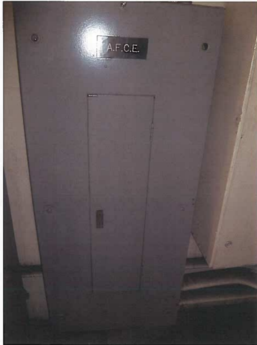
EXISTING PANEL "AFCE"
