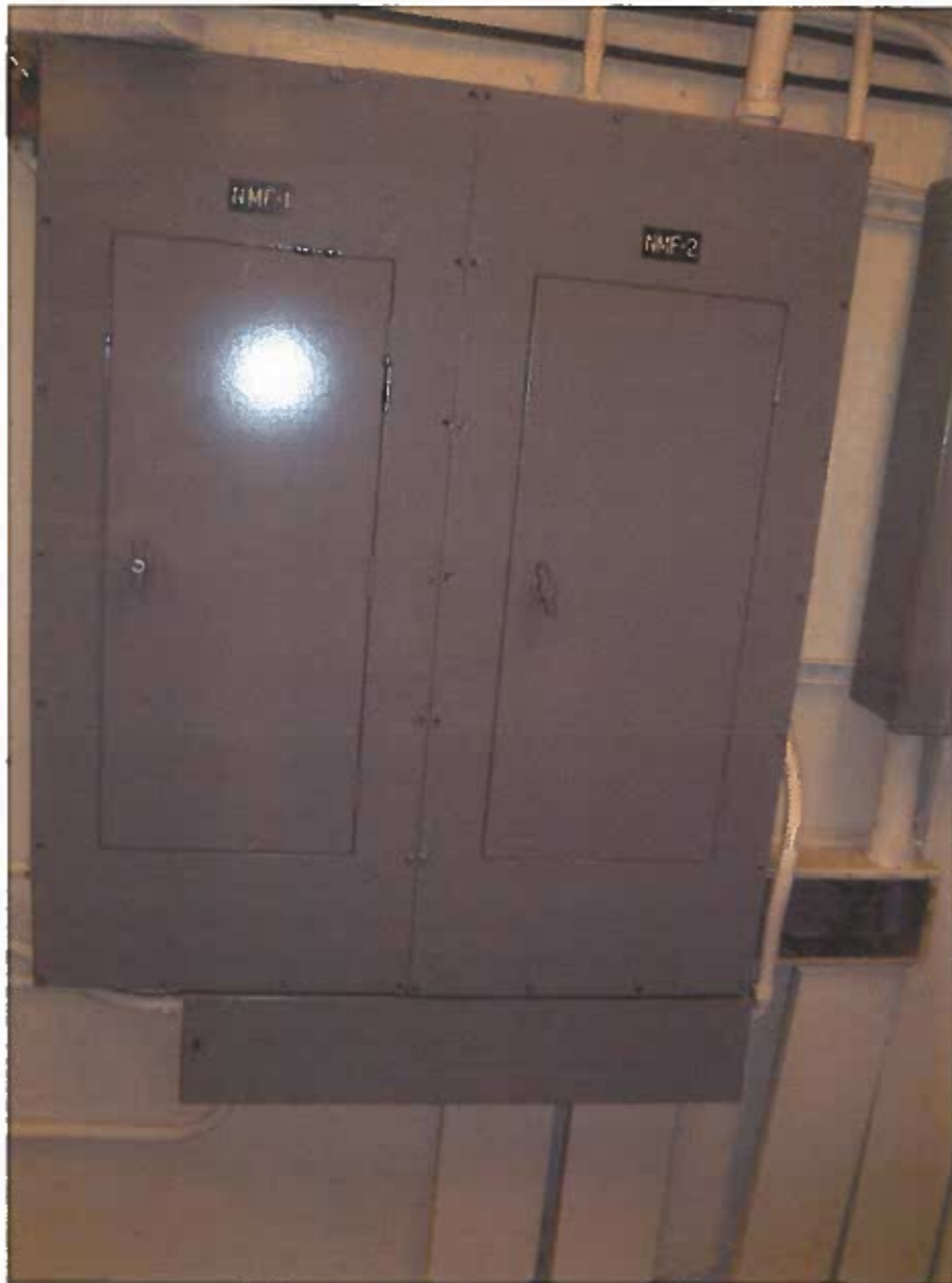
EXISTING PANEL "NMF-2"
