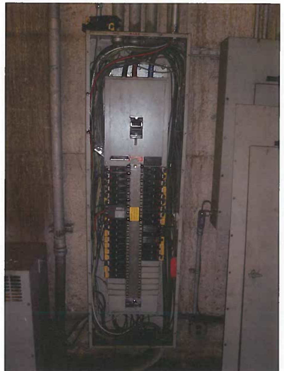
EXISTING PANEL "MSAA"
